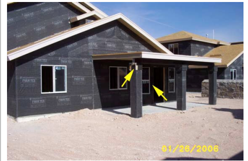
Looking north east @ rear of house – arrows indicate missing column caps and indicates missing stucco lathe 3
