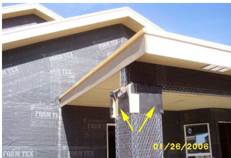
Looking north east @ close up of missing column caps 4
