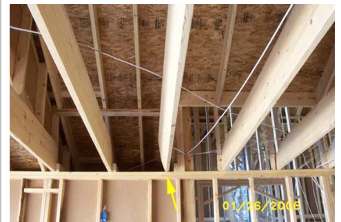
Looking east @ garage interior east side – note arrow points to severe twisting ceiling joist 9
