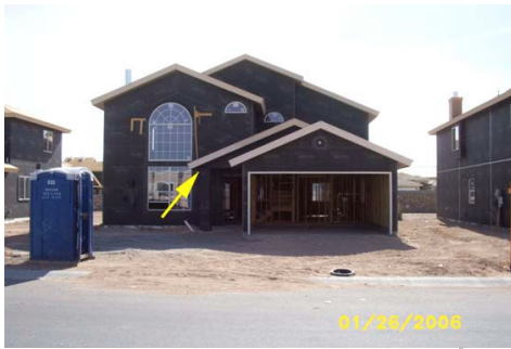
Looking south @ front of house – note arrow indicates missing stucco lathe (mesh) 1
