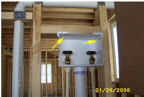
Looking @ washer hook up box – note nails used to anchor in place 10
