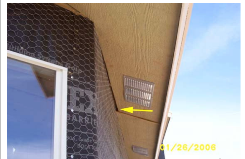
Looking north @ gap along east side soffit 6
