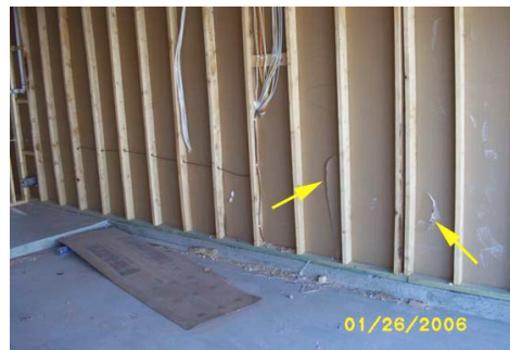
Looking southwest @ garage interior west wall (exterior) sheet rock damage 8
